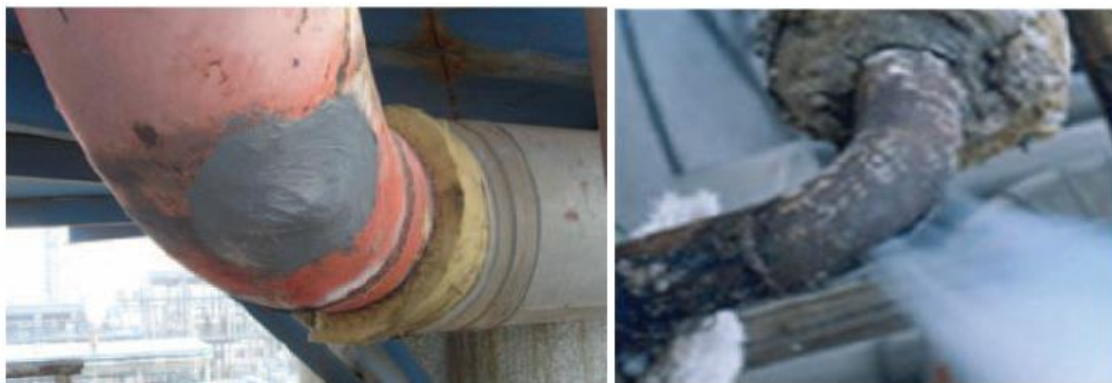
Figure 1: Actual damaged pipelines (a) a failure of bend after repairing; (b) a failure of bend in a gas pipeline
